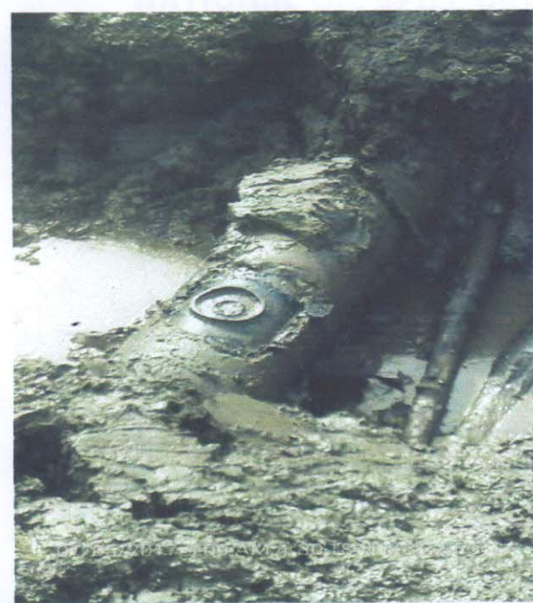
CONE OF PREVIOUSLY REPAIRED WAS CUT OFF
